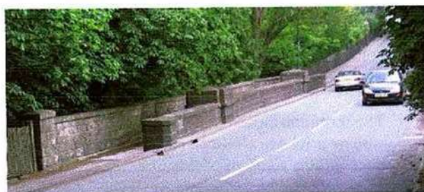
Loose Viaduct, showing the footpath built on its west side in the 1930s
